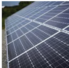
Solar photovoltaic panels
